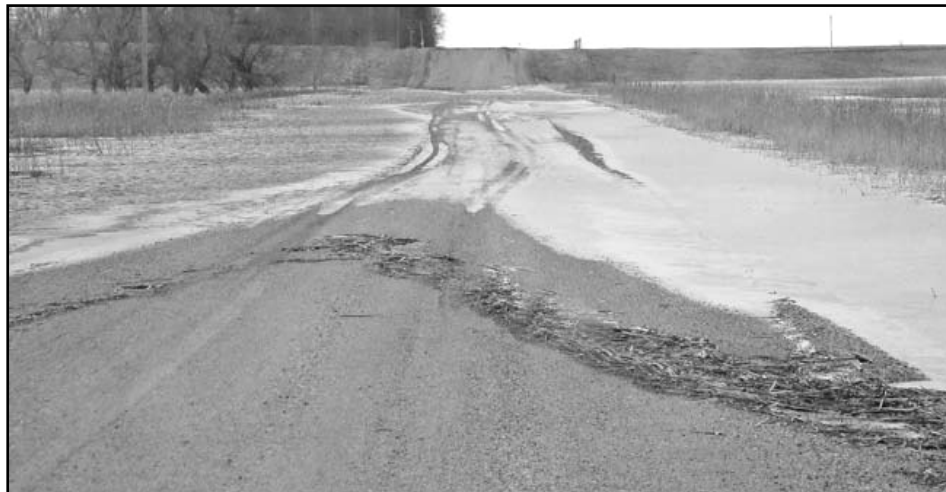
A situation that requires emergency road closure to ensure public safety.
