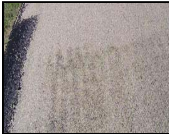
A minimal amount of cover coat aggregate is used in Burleigh County's new chip sealing method.
