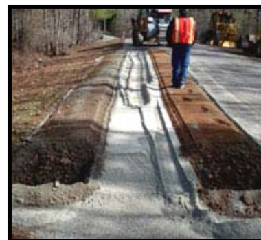
The Asphalt Zipper pulverizes the failed asphalt roadway and mixes it with cement.
