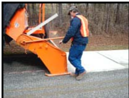
Cement is distributed evenly over the roadway with a modified chip spreader.
