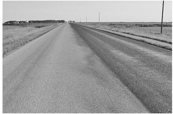
Fog seal completely coats the chip sealed surface and retains stone very well.
