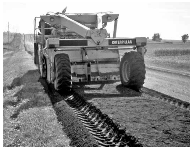
In-place recycling of asphalt surfaces is an option to consider in surface rehabilitation.
