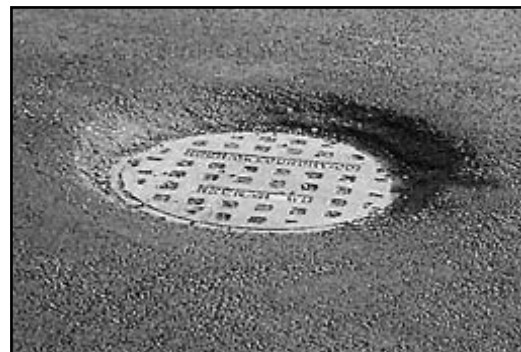
Sunken manhole should have been raised before paving.
