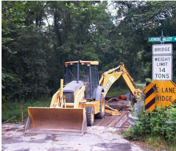
Illustration of a poorly implemented TTC lacking a detour or road closed sign.
